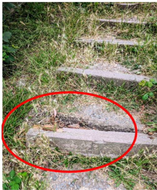
Broken step on landscaped path
